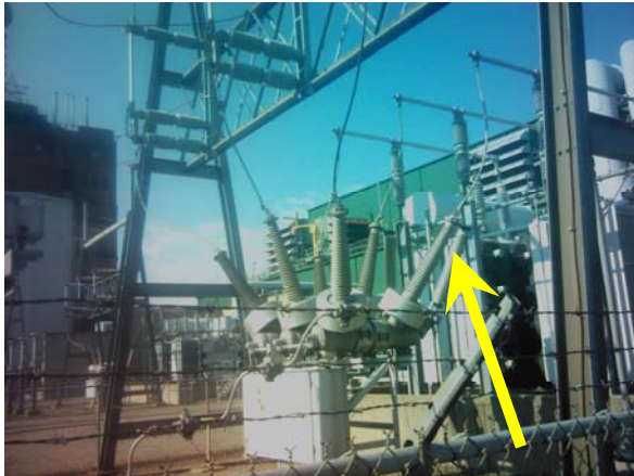
Outdoor High Voltage Substation Gas Turbine Generator No. 2
